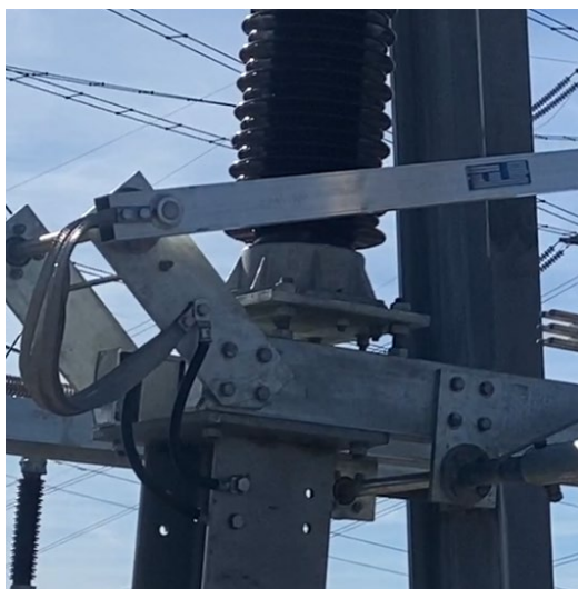
Figure 17.1 Earth switch earthing cables
