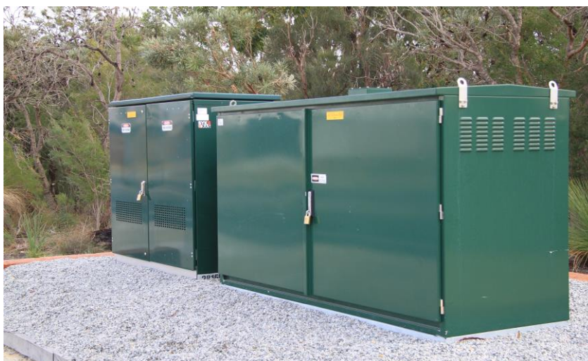
Figure 57: HV outdoor ground mounted switchgear & transformer
