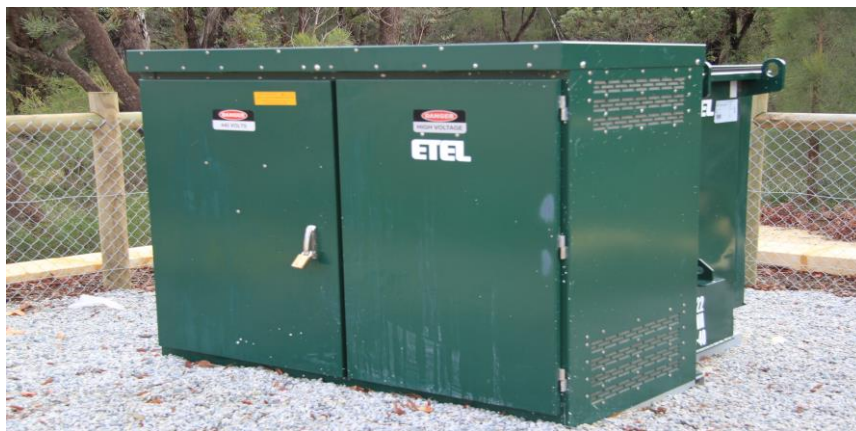
Figure 55: Modular package substation
