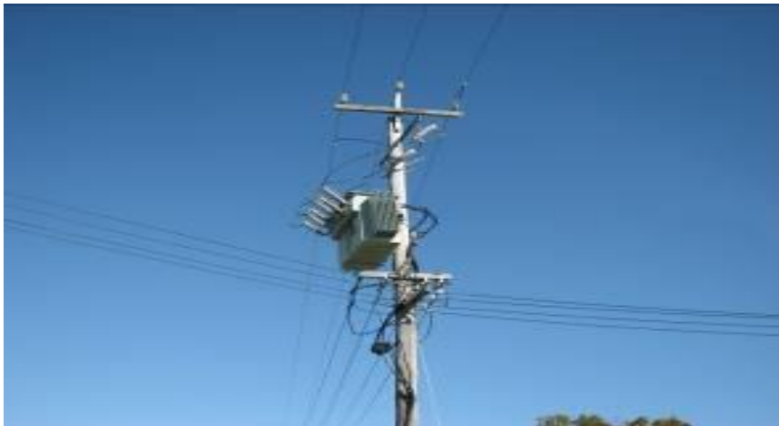
Figure 58: HV outdoor aerial mounted equipment
